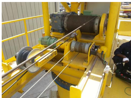
Hoist and travel winches
