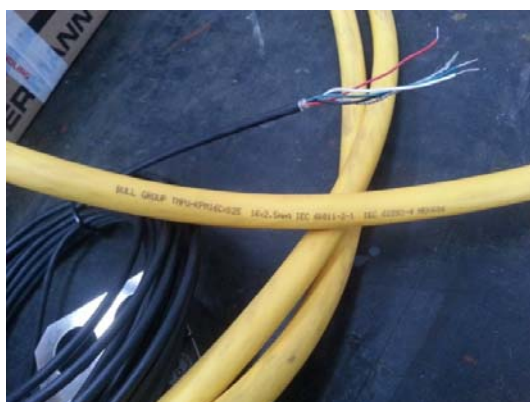
High quality cables
